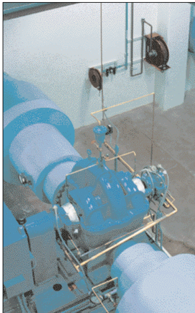
Figure 1. One of four 30 MGD 30 x 24 MAA horizontal pumps operating in the facility.
