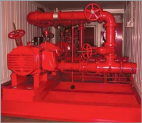
Completed housed unit.
